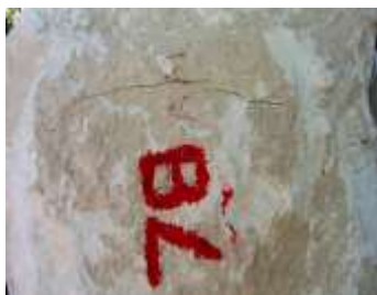
Fig.(6) shows the cracks and microcracks.
